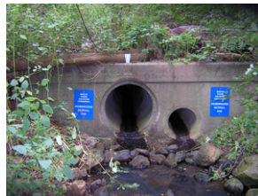
Storm Drain Outfall
