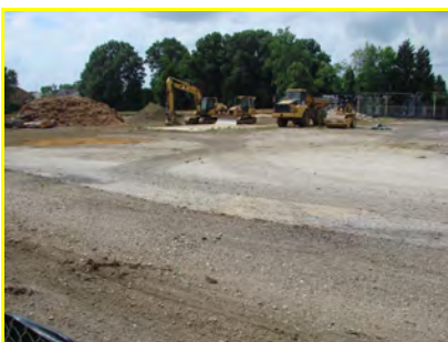
Remnant concrete & other nonerodible surfaces
