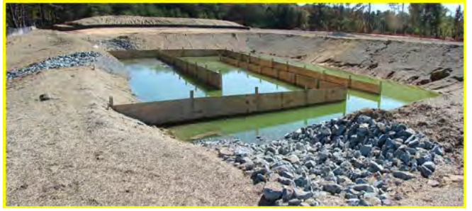
Perimeter Sediment Trap
